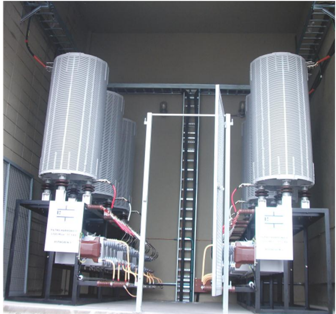
Fig. 15. Filters room, and the two tuned harmonic filters.
